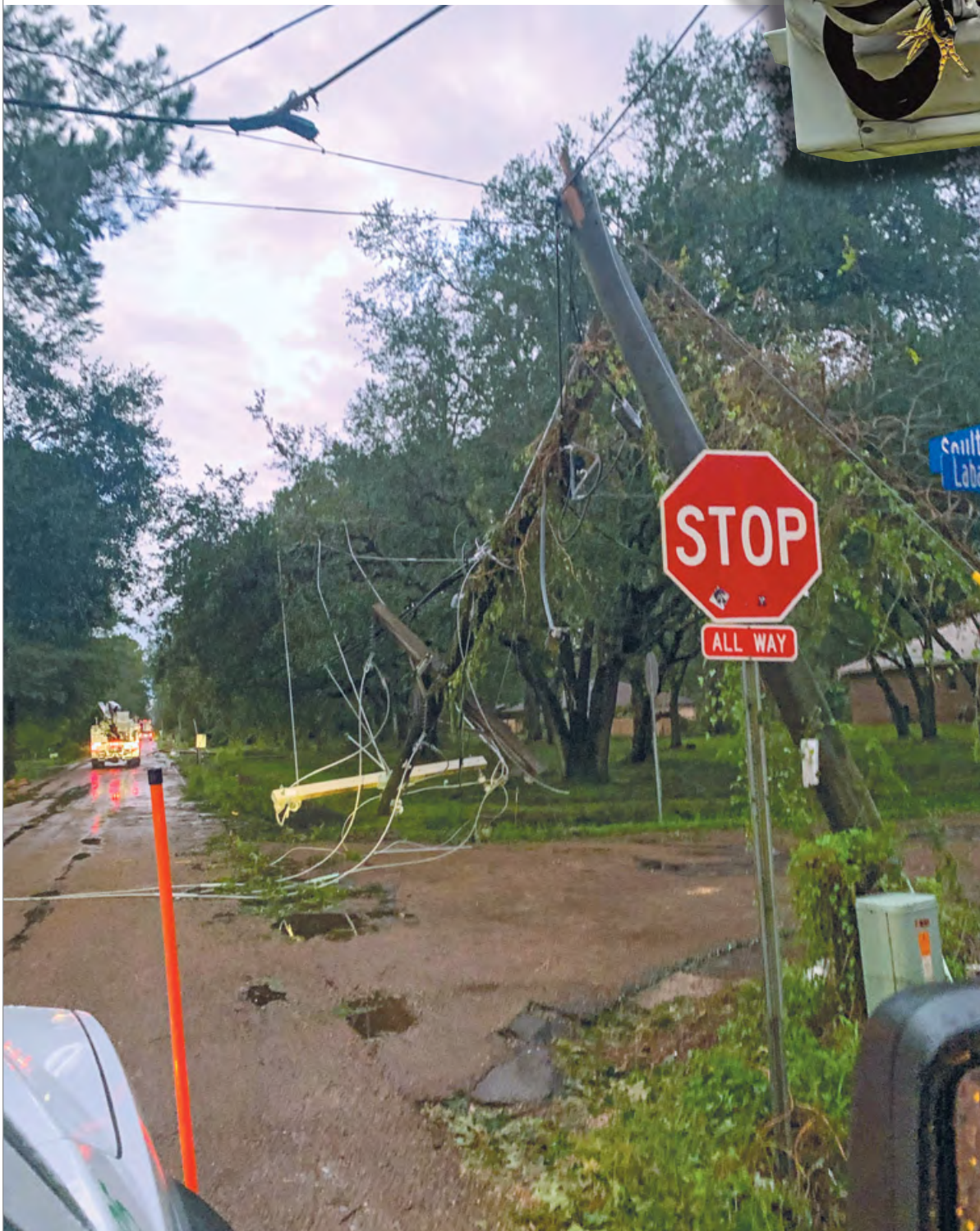
Category 4 Hurricane Ida did more damage to electrical transmission in Louisiana than Katrina and three more recent hurricanes combined, leaving a million people without power and tens of thousands of poles in need of repair or replacement.
