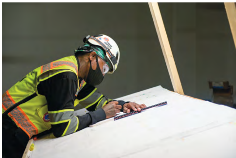
Local 26 member Travis Bennet is foreman on the Ashburn project for Sabey Data Centers, which is part-owned by one of the IBEW's pension plans.
